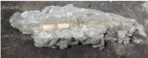
Figure 11: Engagement on bamboo and concrete, observed post failure.
