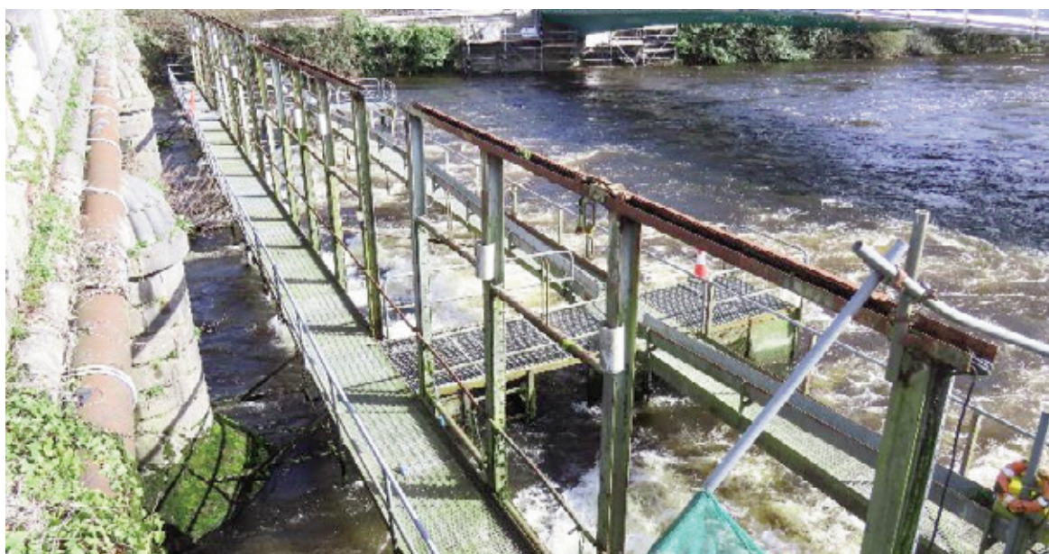
Figure 10: The river-wide obstacle at the Salmon Bridge, viewed from downstream.
