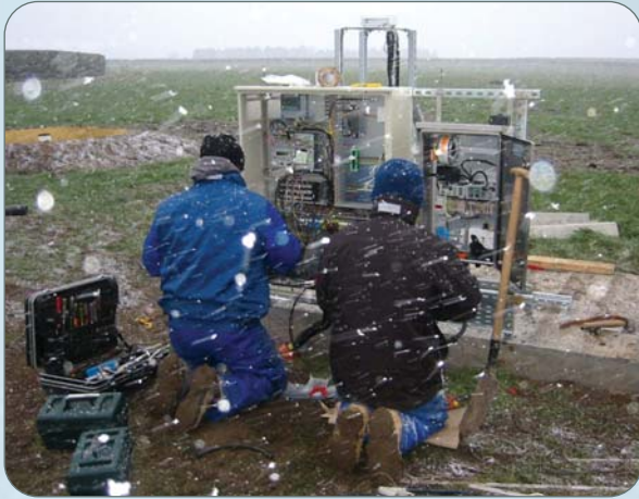
Instruments Unit staff working on installation of new TUCSON station at Grange during a snow shower [February 3rd]
