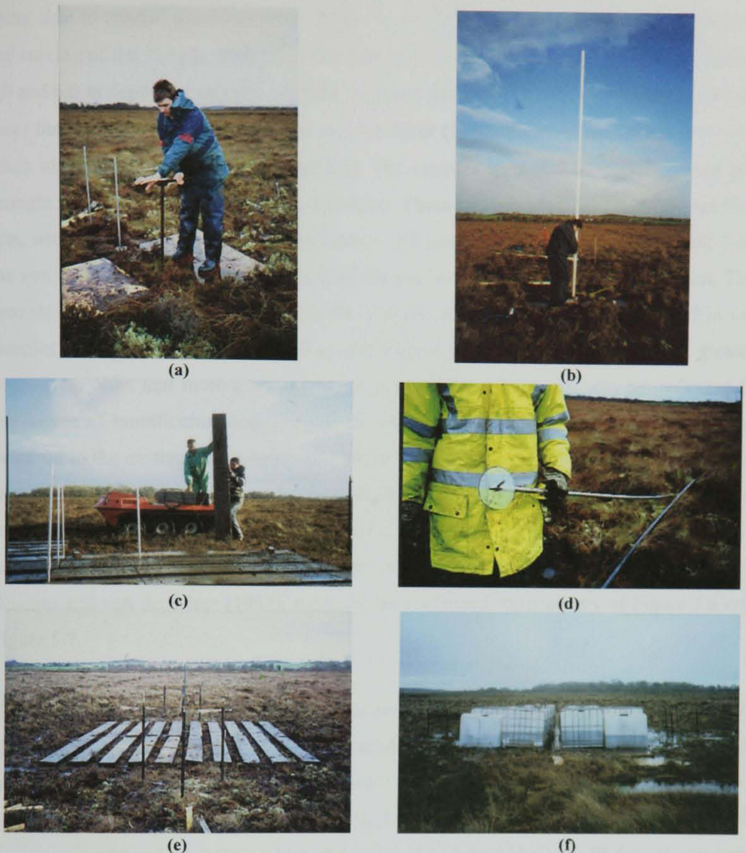
Figure 5.9 (a) Hand-augering holes for settlement plates (b) Inserting benchmarks (c) Placing railway sleepers (d) Settlement plate (e) Test site before the tanks were positioned (f) Test site conditions, March 1999
