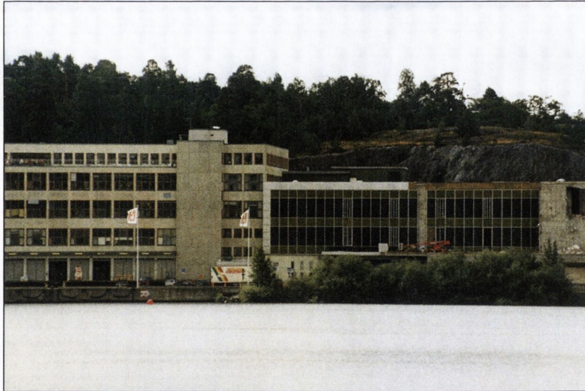
Figure 6.11: Part of the Wine and Spirits Central in Liljeholmen undergoing demolition when the photograph was taken (Negussie, 2001).
