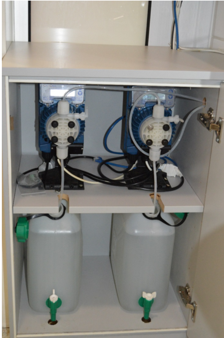
Figure 2.8 Photograph showing the two Tekna dosing pumps and catholyte and anolyte reservoirs located in a lockable cabinet at floor level adjacent to the test washbasin used for automated ECA U-bend decontamination in the present study.
