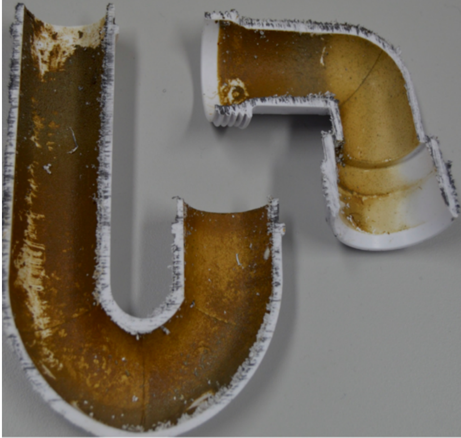
Figure 3.2 Photograph showing a cross-section of a U-bend from one of the control washbasins after the five-week initial study period. Extensive heavily pigmented microbial biofilm is evident throughout the U-bend, including areas above and below where water is retained.
