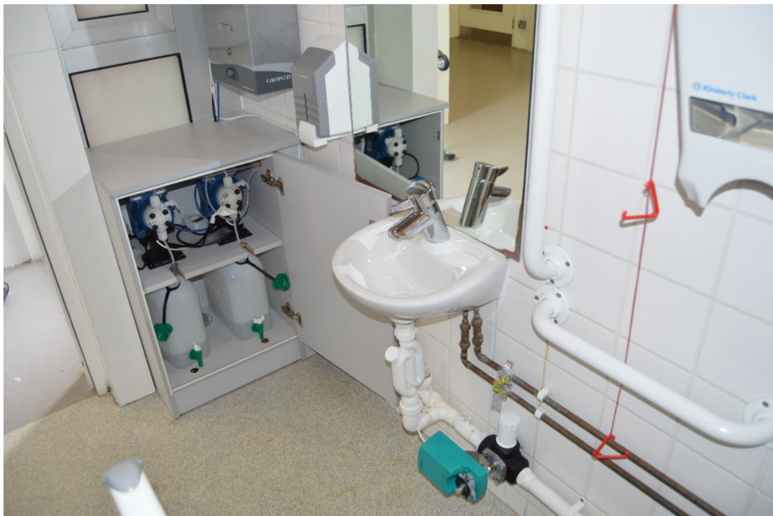
Figure 3.5 Photograph showing the general assembly of the equipment used with the second prototype automated ECA U-bend decontamination system developed in the present study. The system was installed in a first floor staff rest room at DDUH. The process controller is located above the cabinet housing the dosing pumps and ECA reservoirs and is not shown in this picture.
