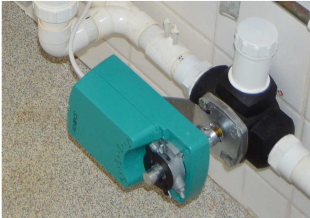
Figure 2.5. Photograph showing the electronic Joventa actuator and Vexve ball valve fitted to the wastewater pipe downstream of the U-bend of the test washbasin used for automated ECA U-bend decontamination. This opens and closes the ball valve in the automated U-bend cleaning and disinfection system developed in the present study.
