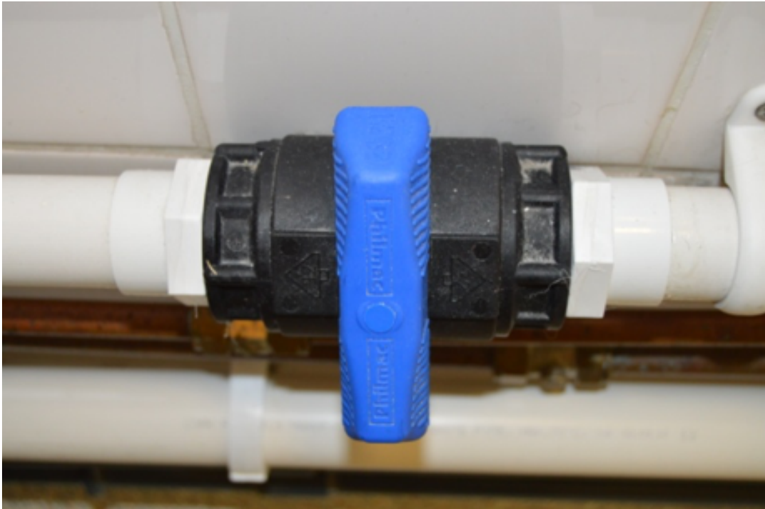
Figure 2.3 Photograph showing an example of one of the manual valves (shown in the closed position) fitted to the wastewater pipework downstream of a washbasin U-bend used in the manual disinfection part of the present study.
