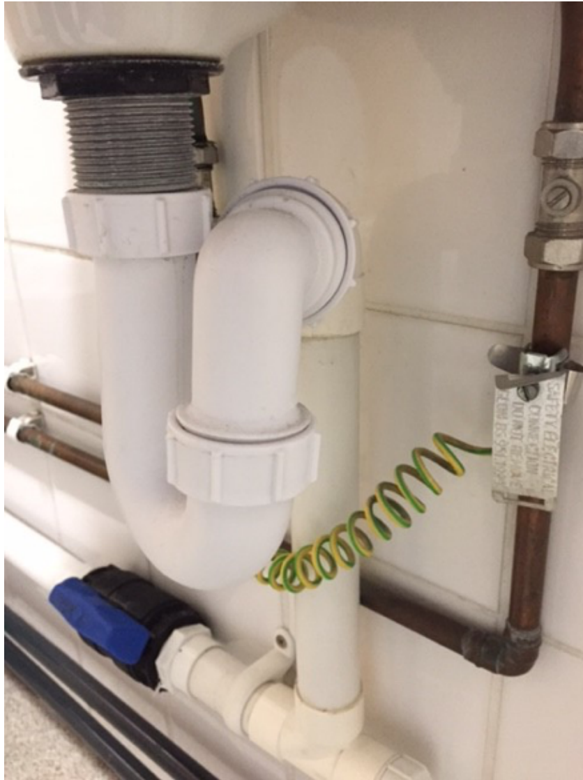
Figure 2.1 Photograph showing a conventional U-bend connected to the underside of a washbasin drain outlet. This washbasin and U-bend was one of three used for manual ECA U-bend decontamination in the initial phase of the study.
