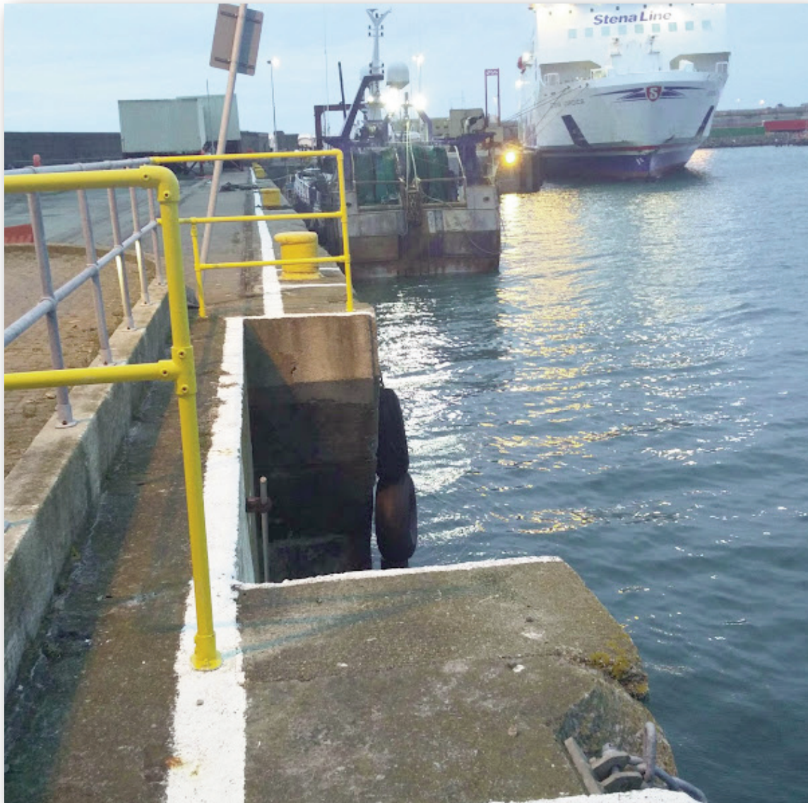
Photograph No. 5. No gangway or safety net were rigged and there is no clear designated access point between the 'MFV Ellie Adhamh' and the quay wall.
