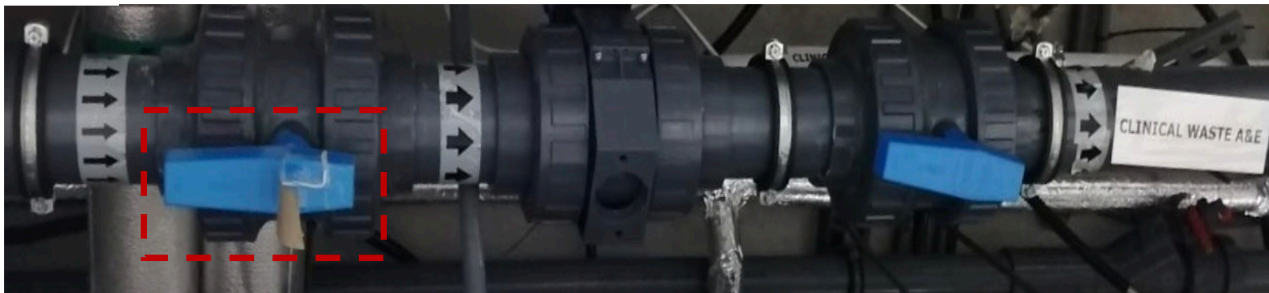
Figure 3.5 Photograph of the common wastewater collection pipe servicing all A&E washbasins located in the DDUH basement beneath the A&E Department. The red dashed box indicates the electronic ball valve fitted to the common wastewater pipe servicing A&E washbasins. Closing this valve permitted backfilling of the wastewater pipes and U-bends of all A&E washbasins with ECA solutions.
