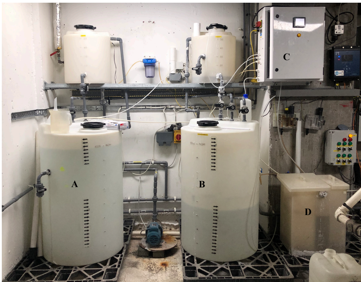
Figure 3.4 A photograph showing the ECA generator and anolyte and catholyte storage tanks used in this study. All were located in the basement of DDUH under the A&E Department. The anolyte (A) and catholyte (B) storage tanks, the ECA generator (C) and the brine solution storage tank (D) are indicated.
