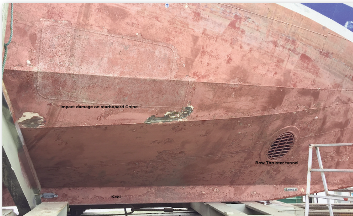
Photograph No. 5 - Starboard Chine damage below the waterline.
