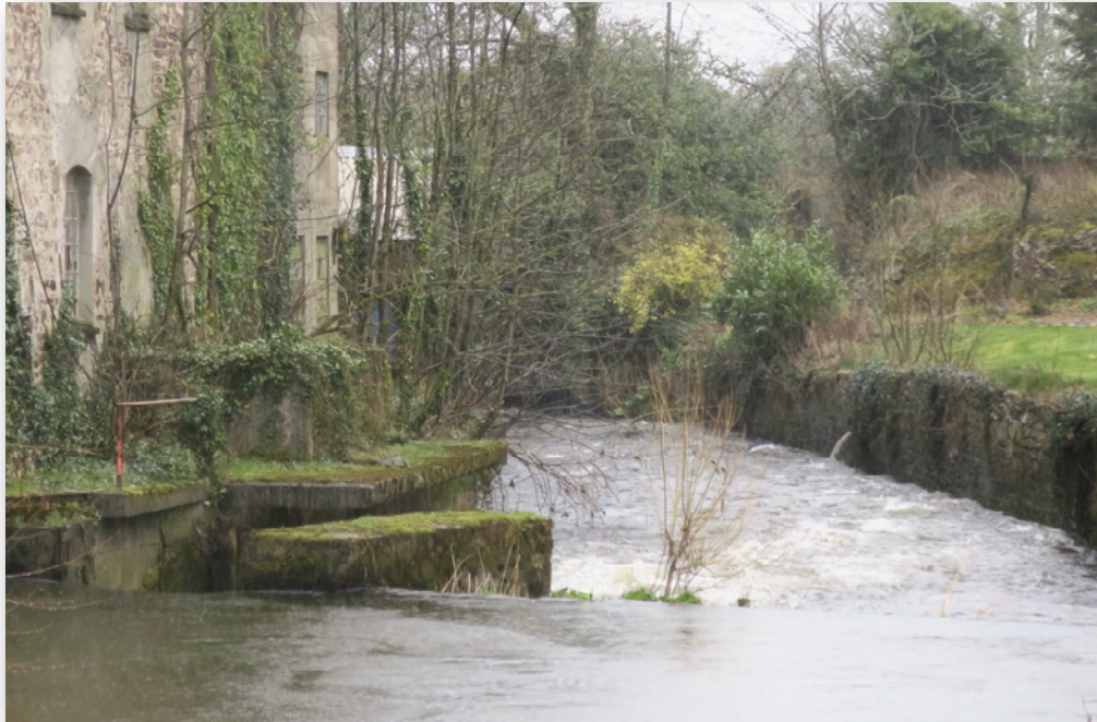
Photograph No. 8: Sluice and weir, sluice on the left-hand side of the photograph.
