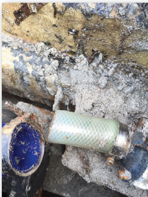
Photograph No.4 - Joints came apart with light pressure.
