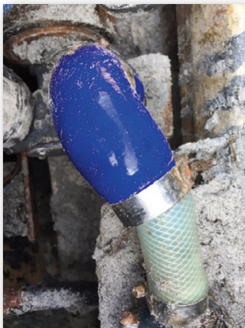
Photograph No.3 - Elbow between oil cooler and water pump.
