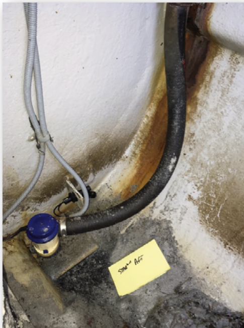
Photograph No.7 - Water ingress in aft starboard compartment.
