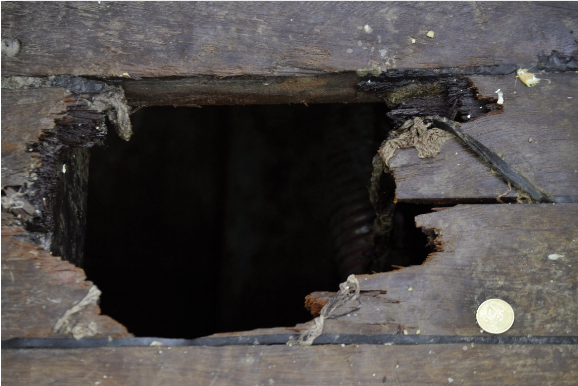
Appendix 7.6 Photograph No. 2 - Hole in Deck
