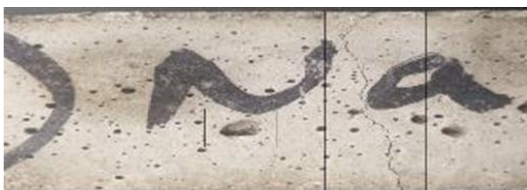
Figure 4 NaOH activated GGBS, 60°C-cured, after salt crystallization cycling showing cracks.
